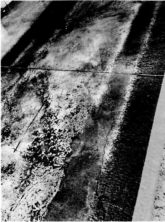
Floor Corrosion and Cracking (Left Bay)
